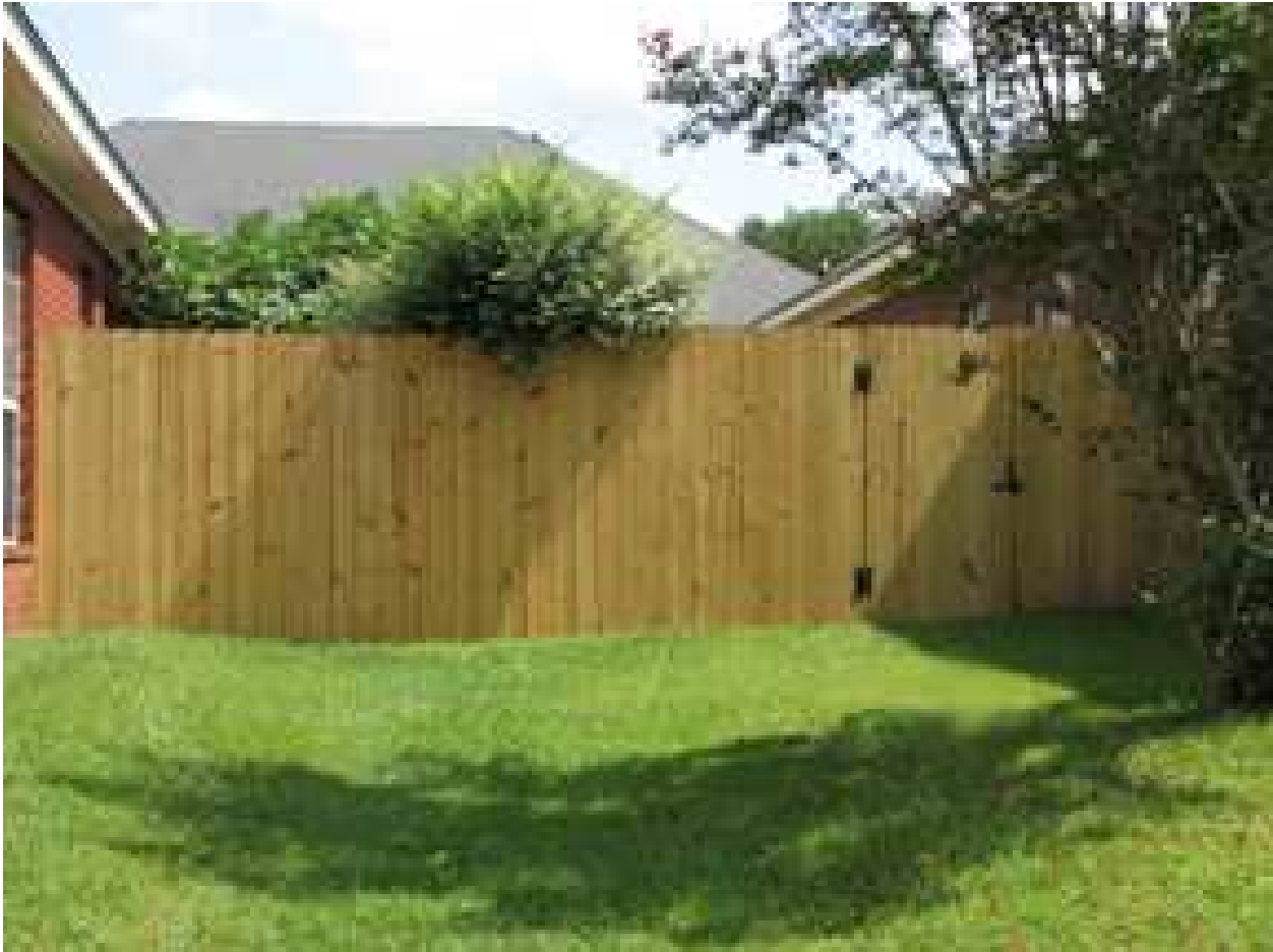
Front fence rebuilt between the Wolfe and Shumacher homes at the corner of South and West
